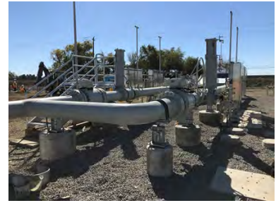
Figure 15 – M&C Complex Station-Above Ground
