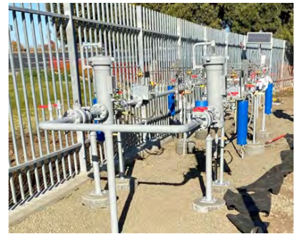
Figure 16 – Large Volume Customer Transmission Station
