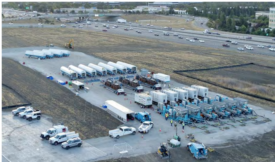
Figure 19 - A Large-scale LNG injection Site in Dublin, CA supporting a planned gas outage.
