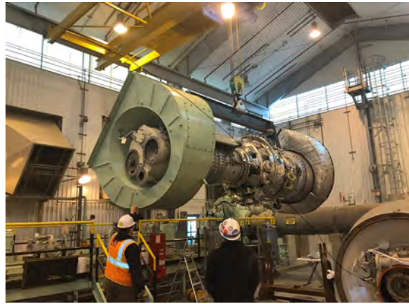
Figure 13 – Delevan Compressor Station Turbine Exchange
